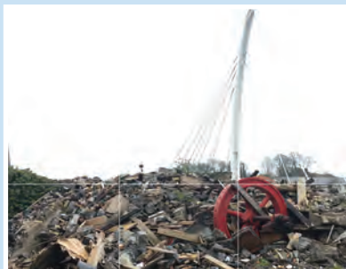
The remnants of a hydro electric wheel in the rubble of a demolished building
